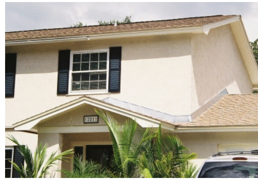
Unacceptable: unpainted flashing and roof drip edge
