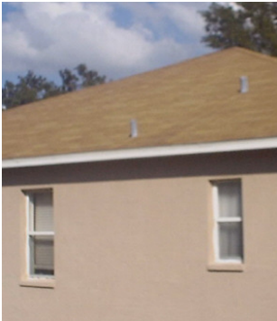
Unacceptable roofing: 20-year non-dimensional shingles. (Shingles are flat and have no shadow or thickness to them)
