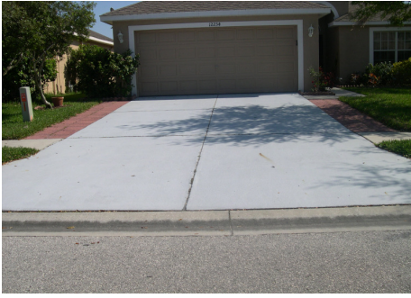
Unacceptable blue stain on driveway
