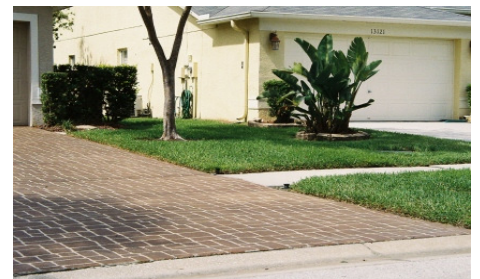
Unacceptable installation: paver material not flush with curb and street sidewalk. The paver material itself is acceptable.
