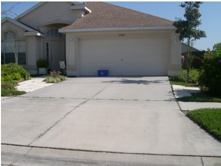
Unacceptable: driveway extension on right hand side is in excess of 2ft
