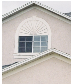
Acceptable: anchor bolts permanently attached to home
